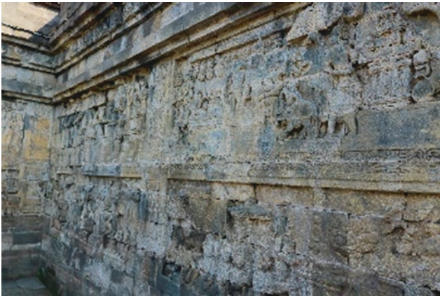
Fig. 8 The condition of the reliefs in Borobudur Temple (Source Authors)
