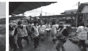
Figure 19 Volunteers from Squad Sukerelawan PAM helped with ensuring the site is safe from debris and waste brought down by the flood at Bukit Lanchong, Puchong
