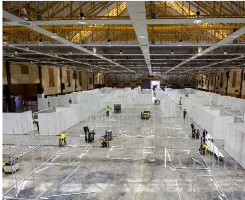
Fig. 4: The transformation work of the main hall (Source: Mardi Corp. Sdn. Bhd.)
